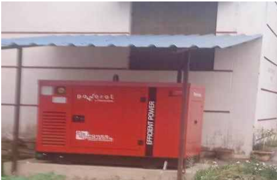
24 Hrs Electricity facilities at KGBV High height Boundary with Watch post
